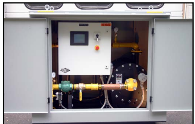
ENGB2 with piping, wiring, and control panel inside outdoor steel transclosure.
